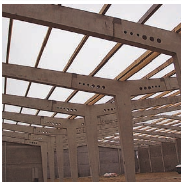
Transport of large components is made easier with small joints - 2 m 3 CRC® JointCast for 20,000 m 2 .
