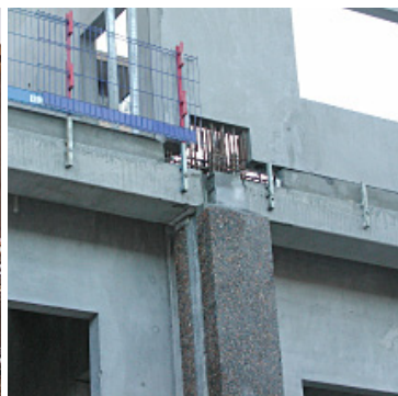
Complicated joints - here 2 beams are joined together in the same spot as a column has to transfer load from a wall.
