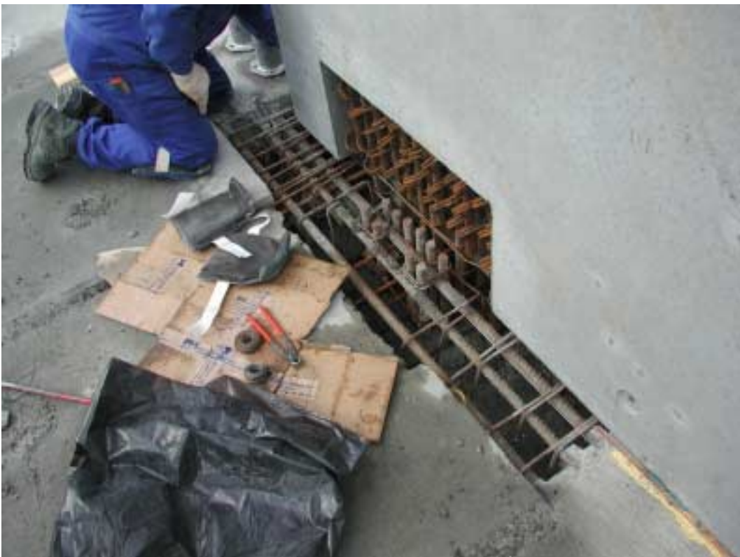
Joint for connection of column and supporting wall at Rigshospitalet, Copenhagen .- and simultaneous beam joint.
