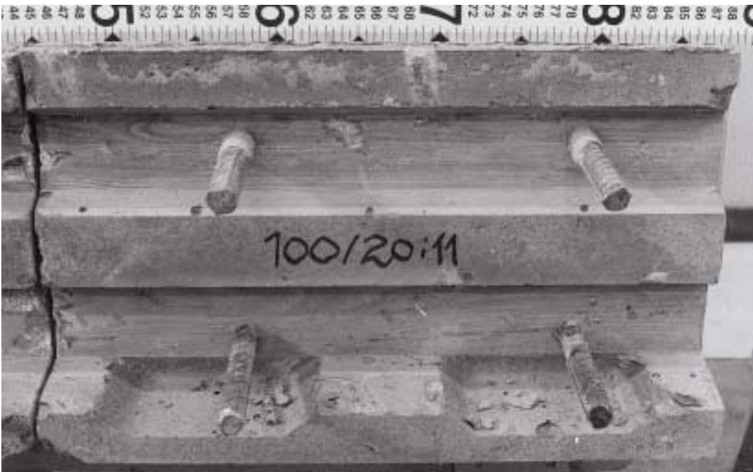
End of bridge slab for the CRC joint. The rebars at the bottom have a 20 mm cover.
