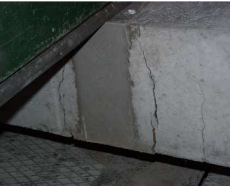
Simple joint with 12 mm bars and a width of 100 mm. The beam fails away from the joint.
