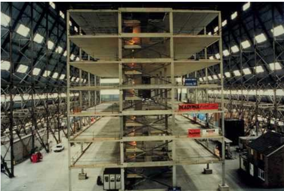
CRC JointCast was used for joining slabs on the top floor of the European Concrete Building Project at Cardington, UK. The staircases were also joined with CRC Jointcast.
