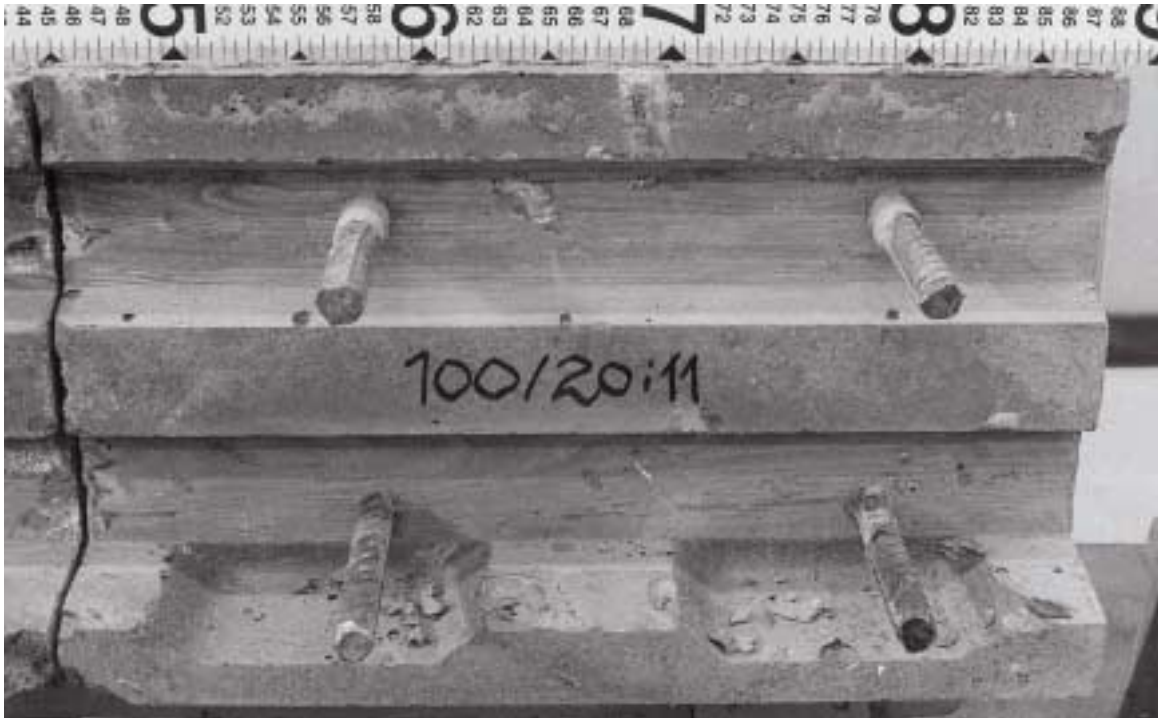
End of bridge slab joint with 20 mm cover to the rebar at the bottom.
