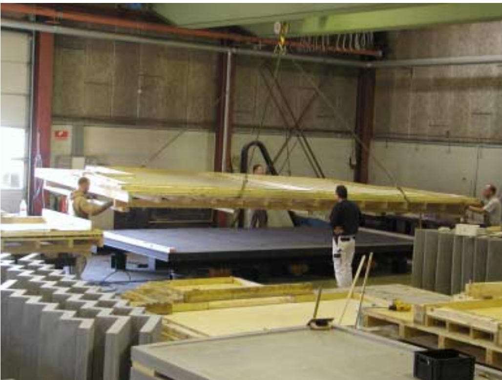
Formwork for balcony slabs being placed on one of the vibration tables at Hi-Con.
