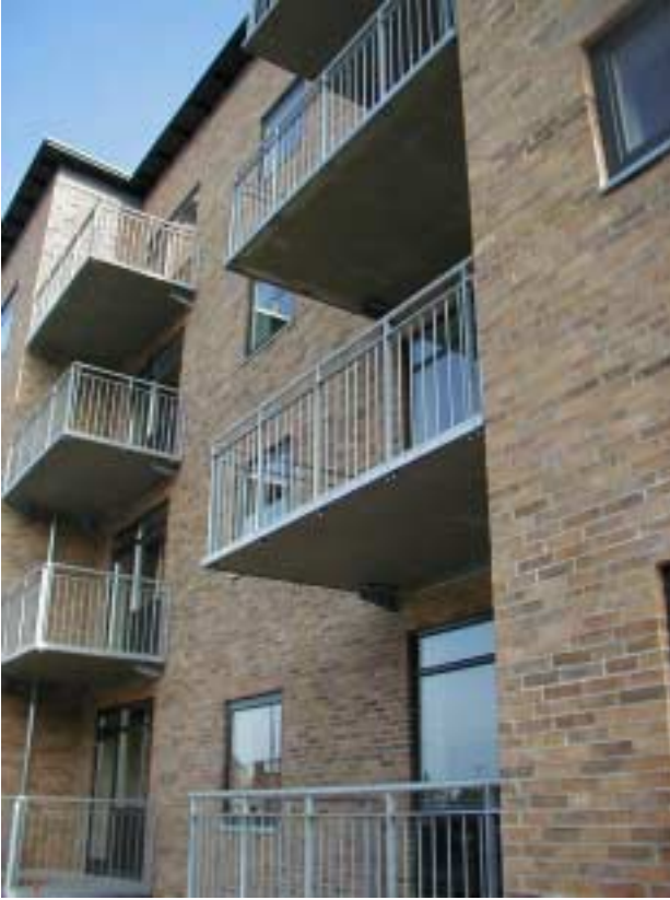
CRC balcony slabs at Vognfjederen, Copenhagen. The slabs are supported at three points and are designed by Arkitektgruppen Århus.
