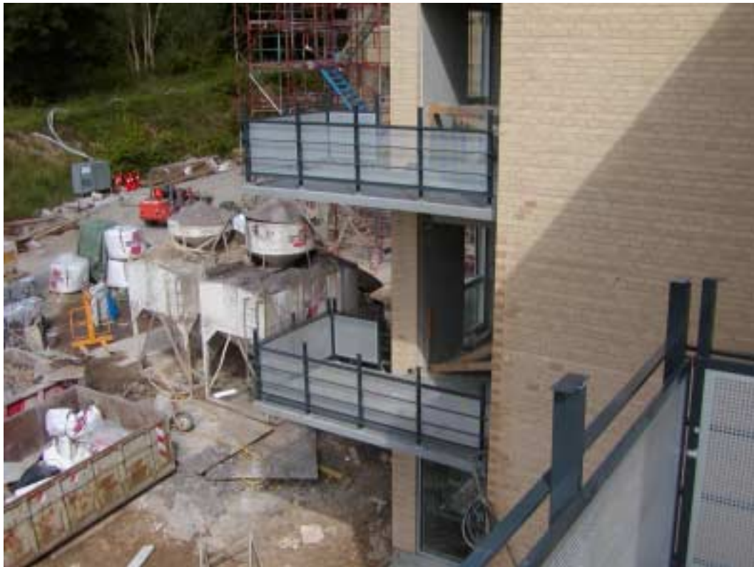
The balcony slabs at Sandegraven, Vejle at different stages of installation. The installation process is quite simple, as the “flaps” are bolted to the floor.
