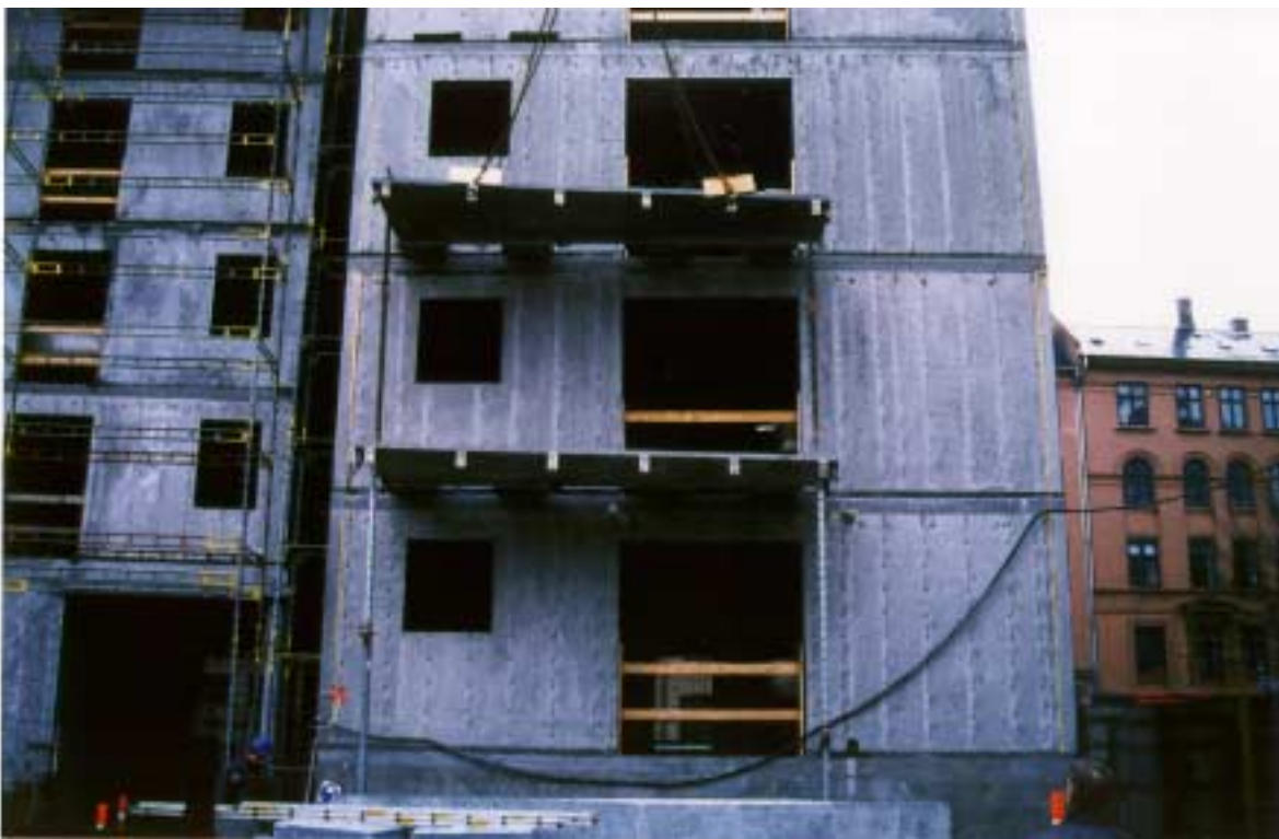
Cantilevered balcony slabs in Nansensgade, Copenhagen being put in place. The slabs are supported by the four “flaps”, that are bolted into the deck. The thickness of the “flaps” is 60 mm to allow room for placing insulation on top and below the “flaps”. Domus architects have designed the balcony slabs.
