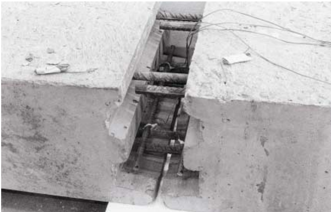
Detail of the joint prior to casting. The rebars were mounted with strain gauges for testing purposes.
