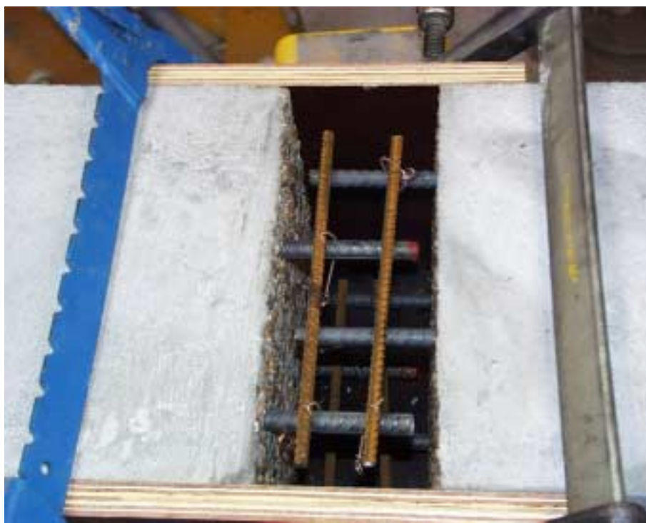
Figure 2 Beam ends with \varnothing 12 mm rebars before the joint is cast with CRC JointCast.
